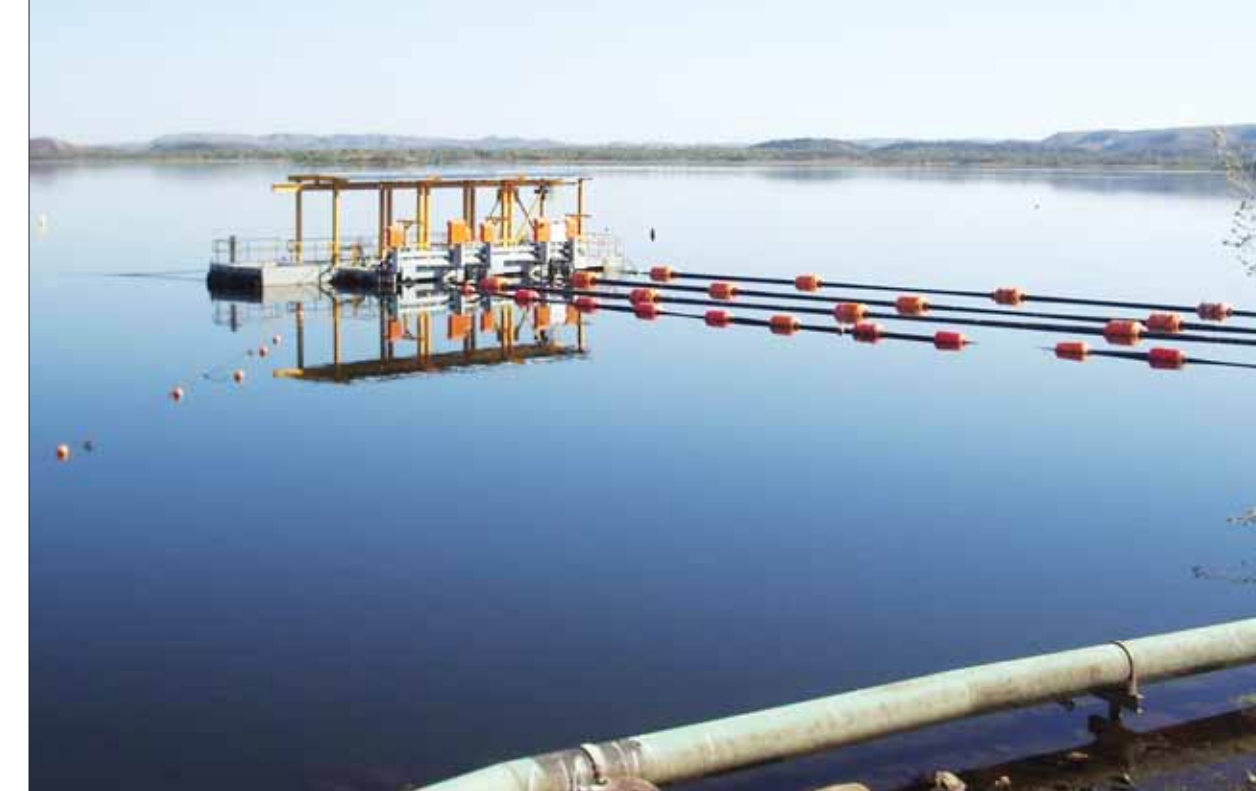
Lake Moondarra is the region's principal water storage area: pictured is Lake Moondarra Pontoon Pump Station which takes water from the lake and sends it to Clear Water Lagoon.
